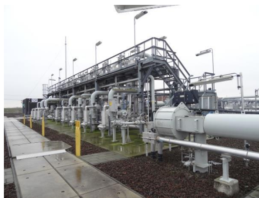
foto 2: Gas metering/ Scrap Area
