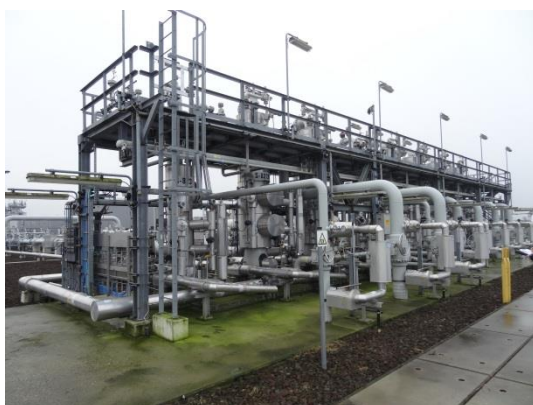
foto 1: Gas metering/ Scrap Area
