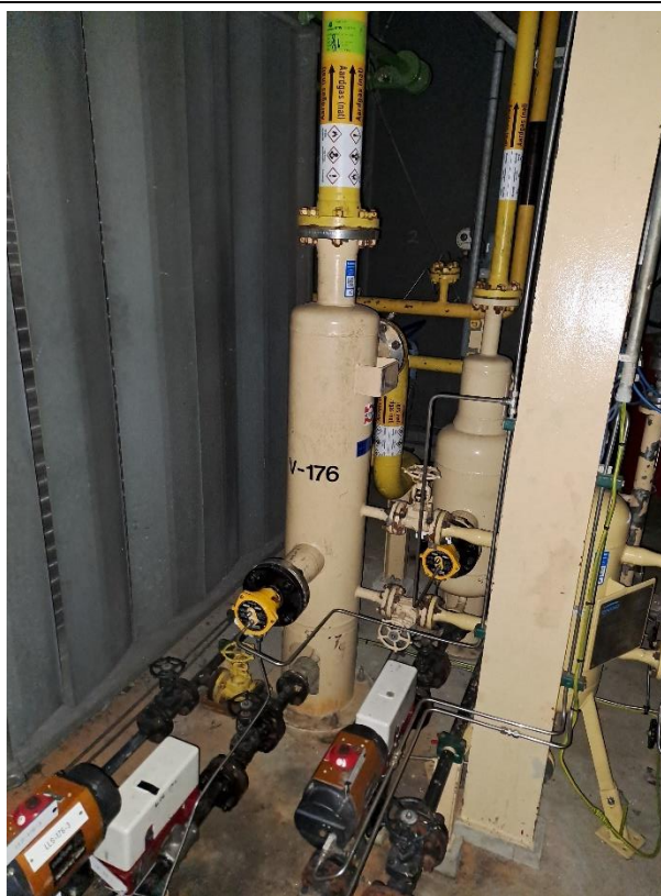
Objectnr. 12 V-176 1st stage discharge scrubber
