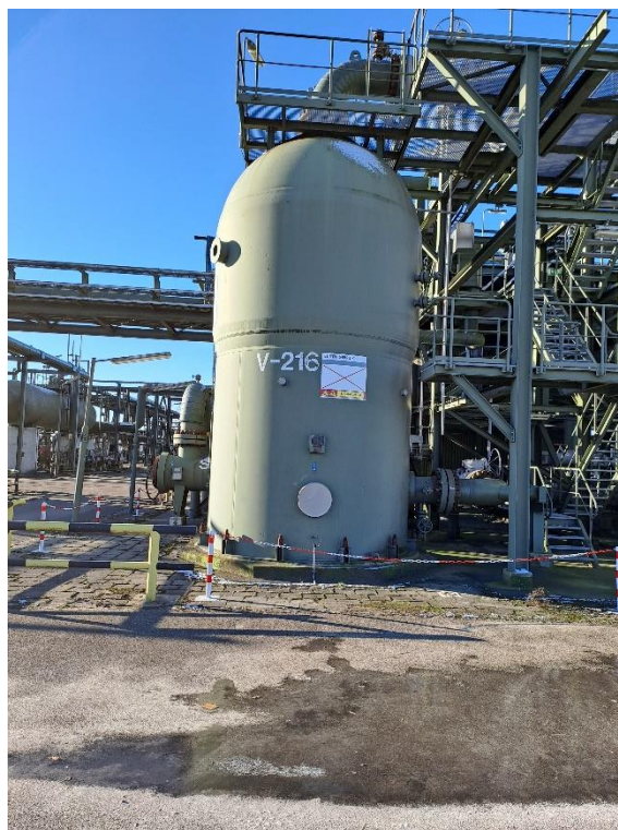
Objectnr. 91 S-216 Mercury removal unit
