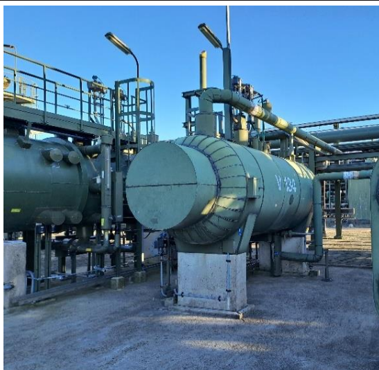
Objectnr. 10 V-134 Condensate stabilization vessel
