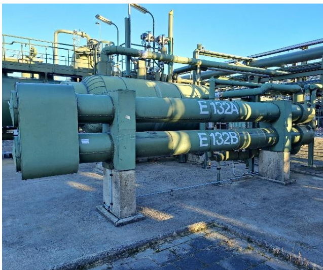
Objectnr. 18 E-132A/B Condensate/Condensate heat exchanger
