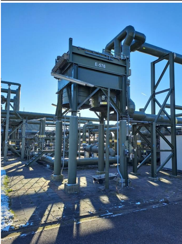
Objectnr. 80 E-576 Discharge gas cooler
