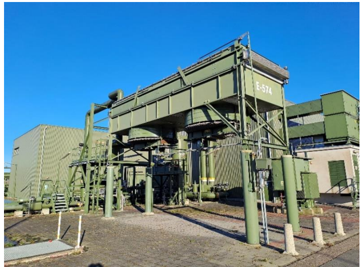
Objectnr. 79 E-574 Inlet gas cooler
