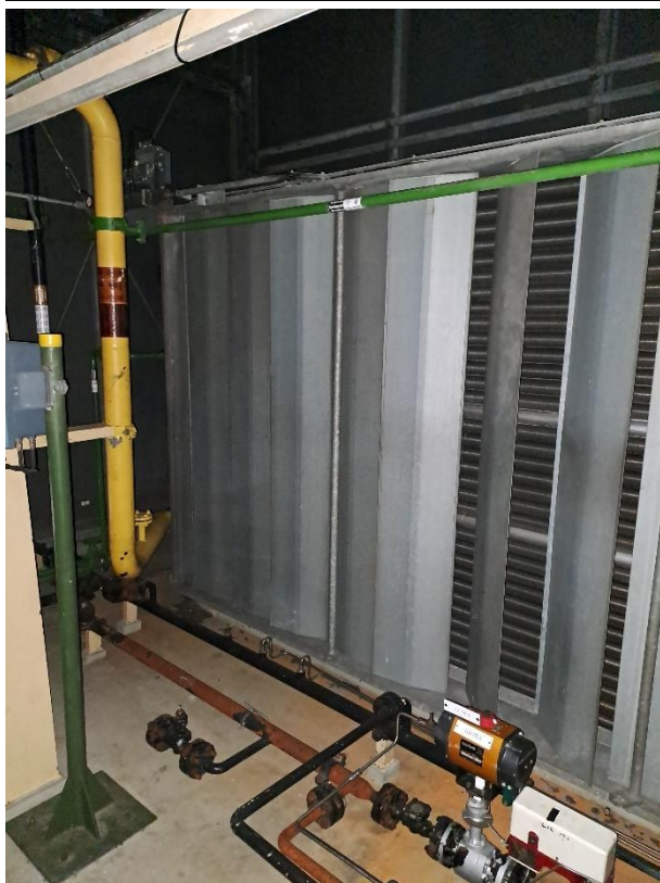
Objectnr. 20 E-175 1st stage discharge cooler
