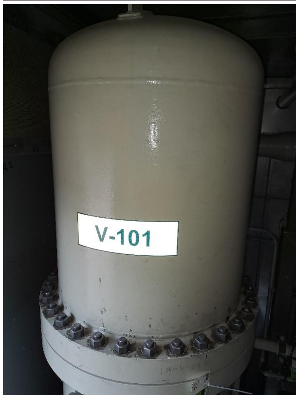
Objectnr. 82 V-101 Inlet scrubber
