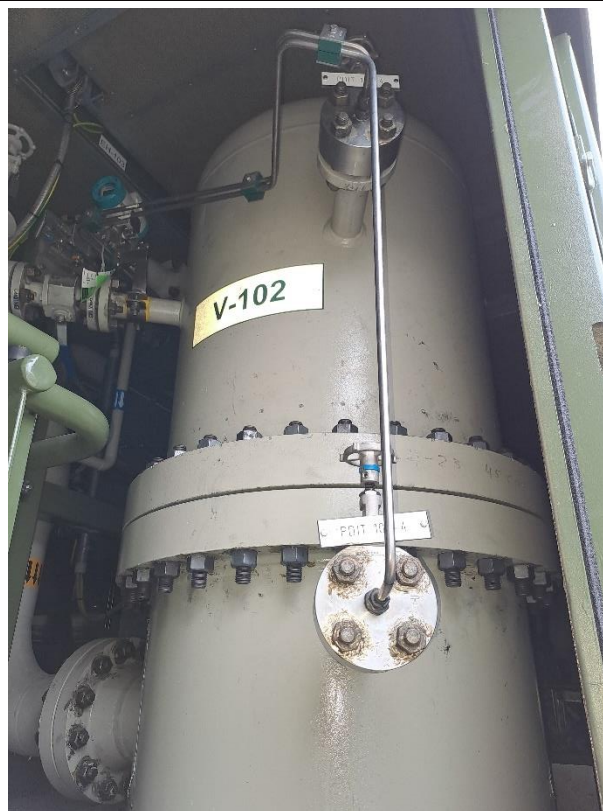
Objectnr. 83 V-102 Inlet scrubber
