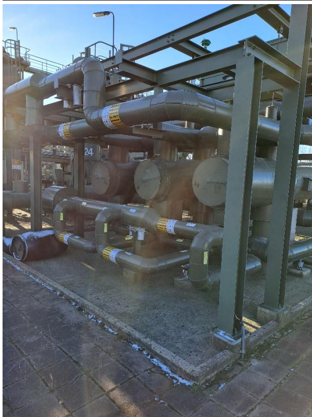
Objectnr. 16 E-121 Gas/Gas heat exchanger
