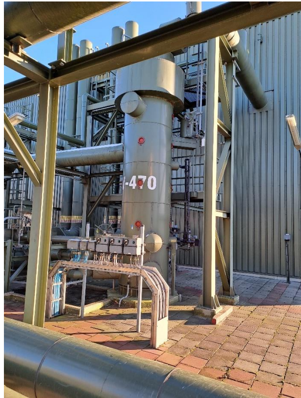
Objectnr. 71 V-470 Inlet scrubber
