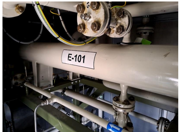
Objectnr. 85 E-101 Inlet gas cooler
