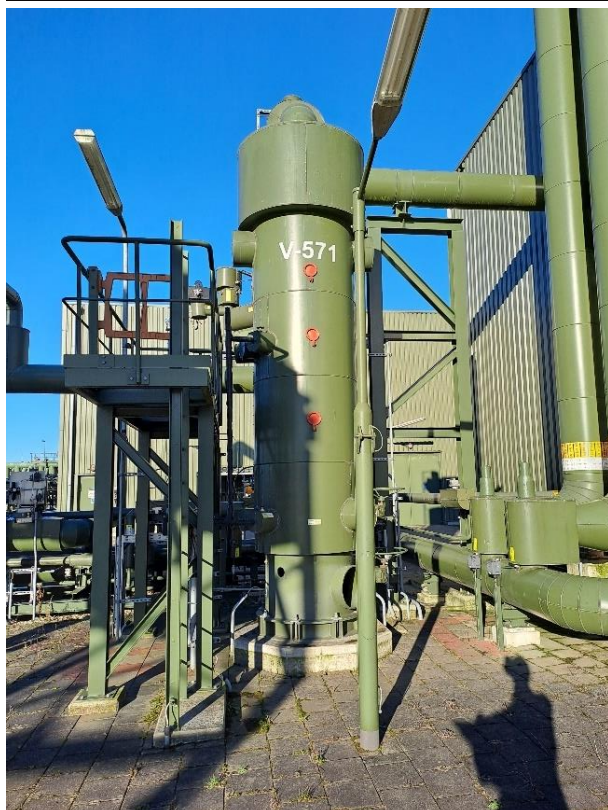
Objectnr. 76 V-571 Inlet scrubber
