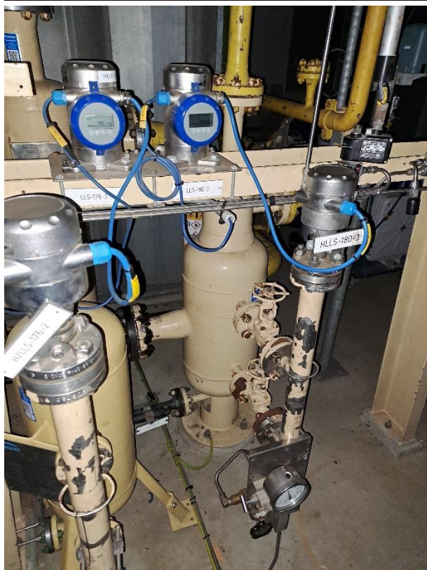
Objectnr. 13 V-180 2nd stage discharge scrubber
