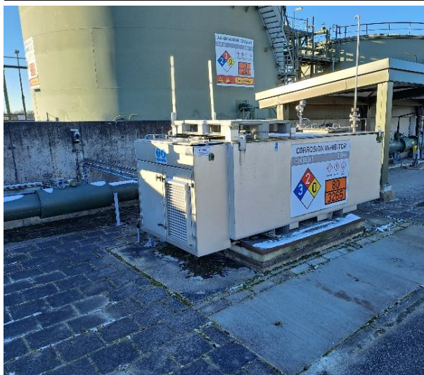
Objectnr. 48 P-90-1 Corrosie inhibitor pump
